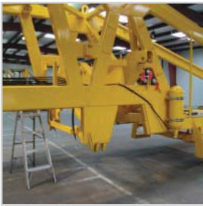
New hoses and accumulators
