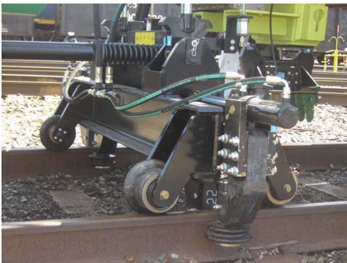
Rail jacks raise the rail while the gripper assembly inserts or removes the tie.
