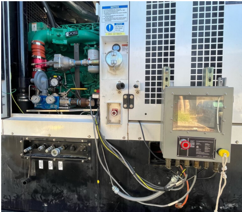
GSSI, FM50, and AFM4 installed on Cummins QSX15
